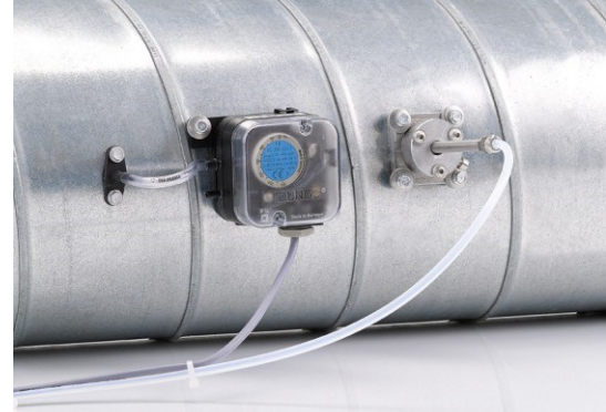
Differential pressure switch 24 VDC and DEBETEK nozzle system on a supply air duct
